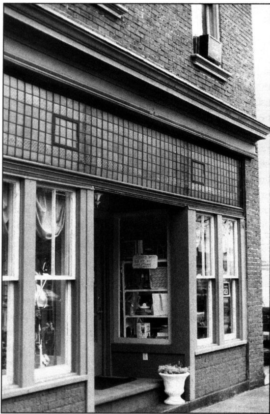
Many prismatic glass installations from the early twentieth century, such this one in Selinsgrove, Pa., combined tile patterns for a striking visual effect.
